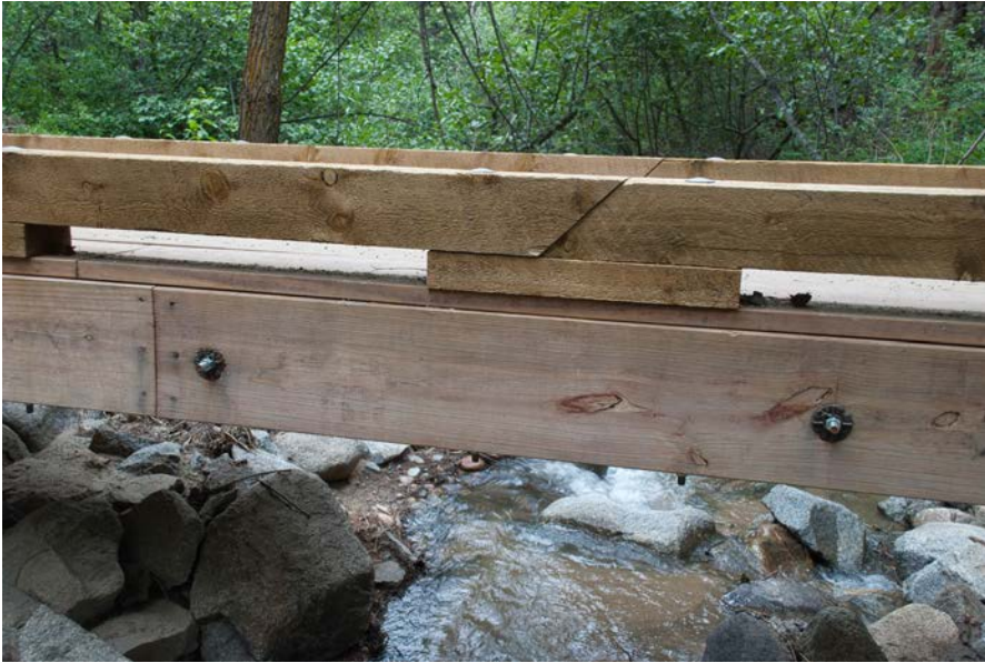
Detail of diagonal splice in timber bull rail and butt-end splice in the bolt-laminated slab.
