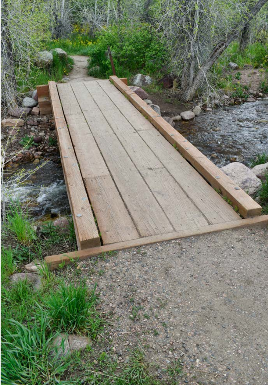
Wearing surface (tread) boards are laid between the toe rails, largely blocking the drainage holes under the toe rail. This placement makes the bridge profile thinner to floodwaters but less visually interesting than the Fourmile Creek bridge. Wear surface boards are standard 2×12s.
