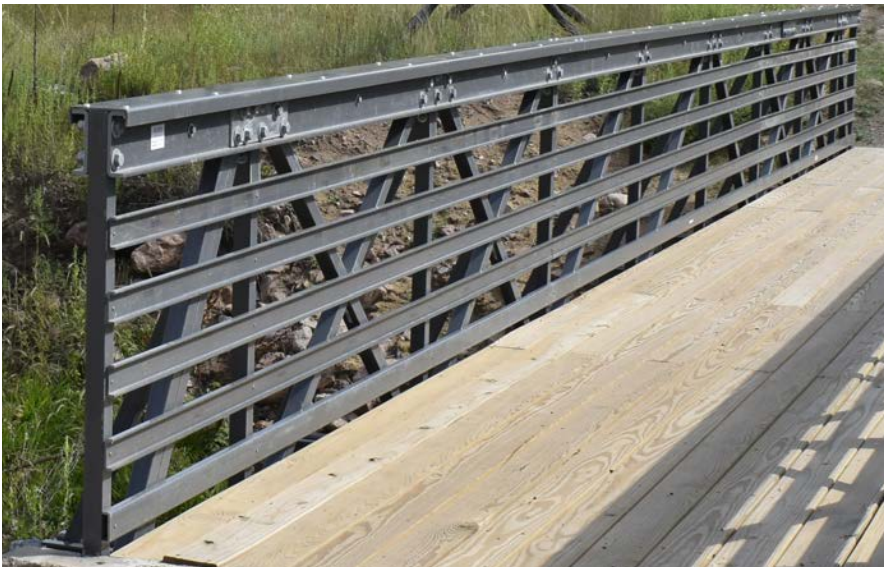
FRC bridge with standard FRC mid-rails (the narrower safety railings between the top chord and the deck) looks and feels like a lot of plastic polymer.
