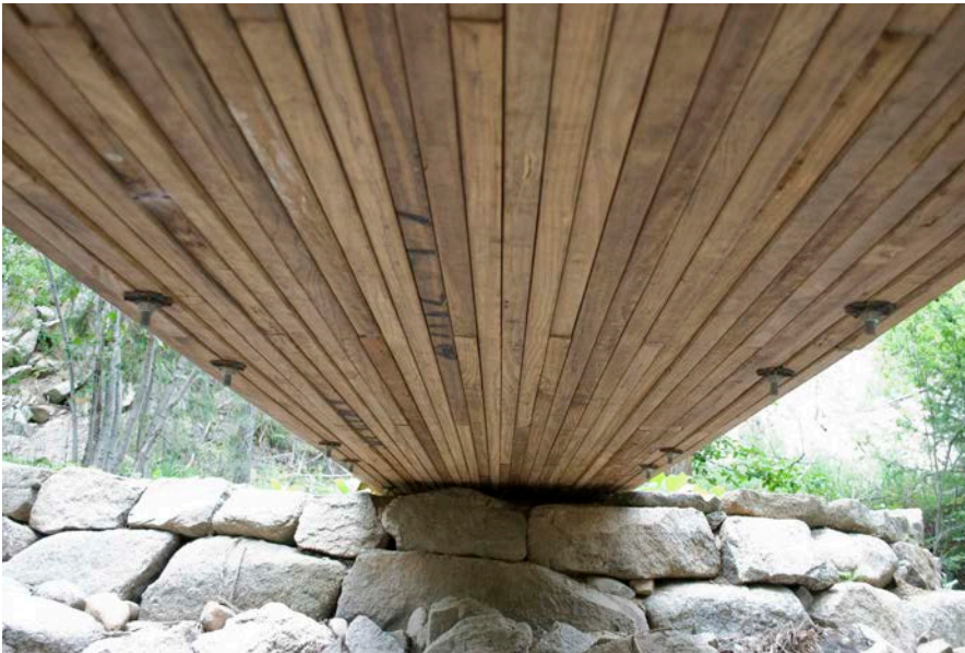
Underside shows that there are no gaps between 20-foot-long standard 2×12s. Butt splices are staggered. Bull rails are attached with long zinc-plated bolts with wide pan heads on top of the bull rail and 2-inch ogee washers and nuts below deck.
