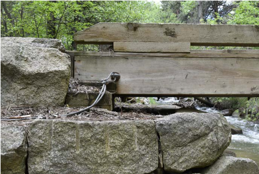
Sills are stacked 2×12s resting on compacted fill behind the stone abutment. The anchor cable and its eyelet on the end of one of the all-thread rods are visible.
