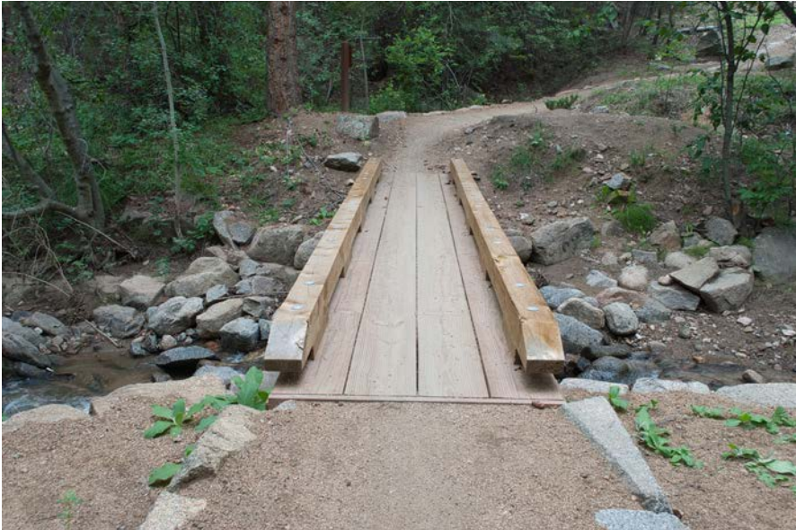
2013—before flood: Initial bridge location in winter. Compare the large tree to the left of the far end of the bridge to which the bridge is cabled and the right side of the far side abutment to the “2015—after flood” photo at right.
