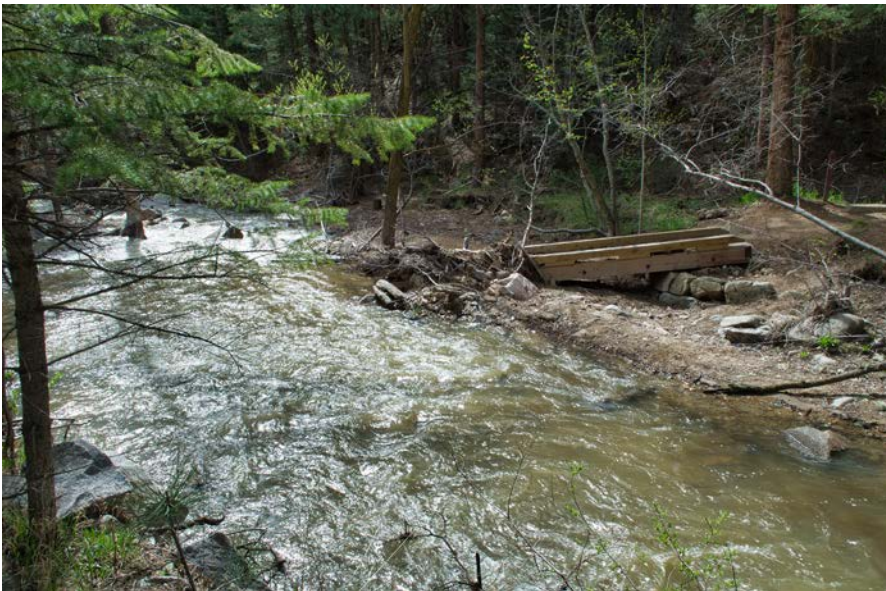
2015—after flood: A powerful flood occurred. New channel is far wider than before and no longer under the bridge. Just over half of the bridge is visible; the remainder is buried under debris.
