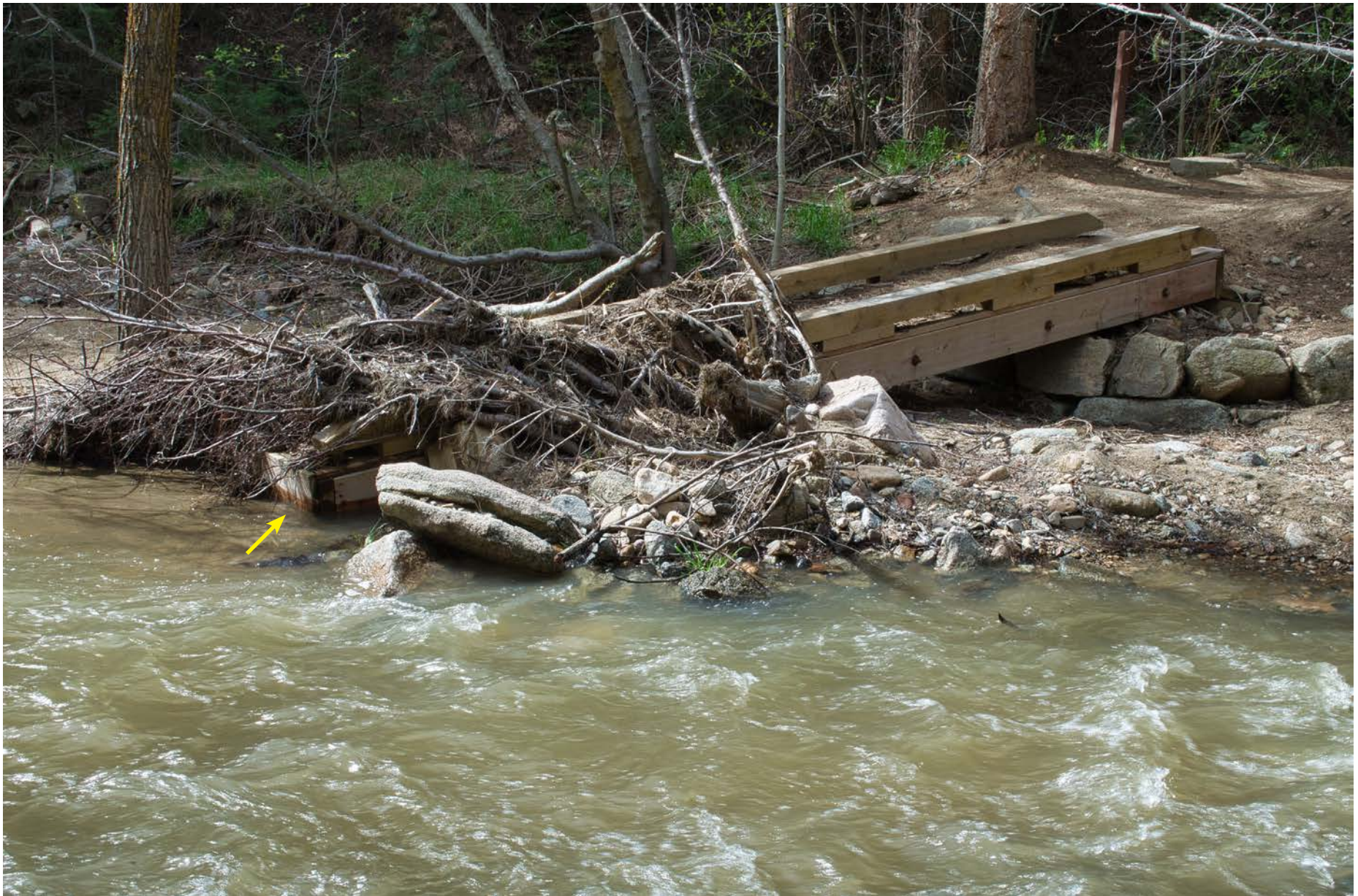
The near end of the bridge is barely visible at the water's edge beneath flood debris (see yellow arrow). Note the doubled end cap. While one dry-laid stone abutment was destroyed and washed away, the bridge itself is not damaged despite the powerful flood.
