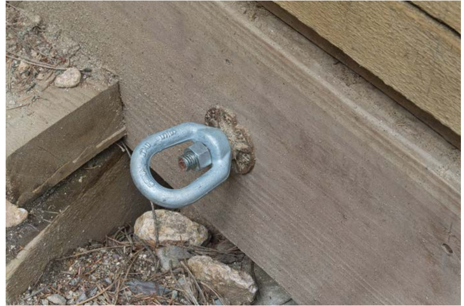
Eyelet and ogee washer bolted at the end of an all-thread rod that extends through the entire deck slab.
