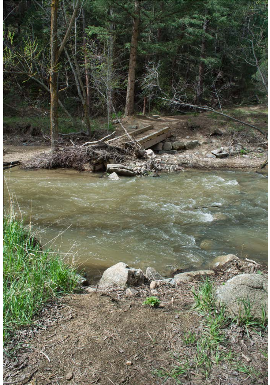
2015—after flood: Bridge in the background after a flood cut an entirely new stream channel on the near side of the bridge. The far end of the bridge is still on its original abutment (compare to “before” view).
