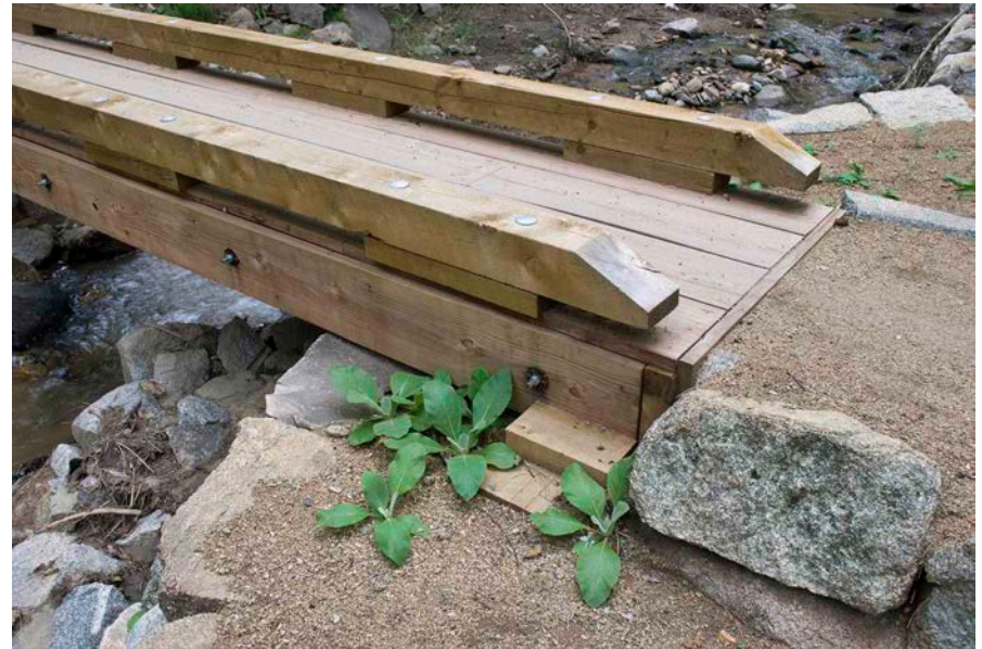
All wood in the superstructure, sills, end caps, and wearing surface (tread) are standard pressure-treated 2×12s. Only the bull rail and 2×6 spacers are full-dimension, rough-sawn, pressure-treated timber.
