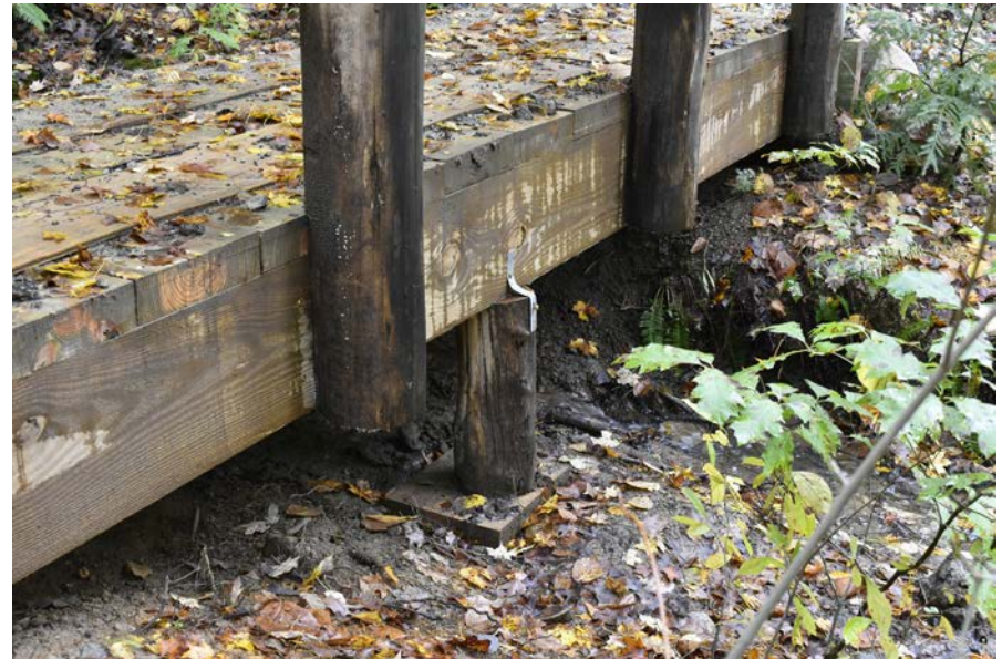
A temporary prop under the center of a short, light-duty, pedestrian stringer bridge enables trail equipment, including excavators and power wheelbarrows fully loaded with trail tread surfacing mix, to safely cross the bridge. The prop was screwed to the stringer to anchor it. Plywood was also tacked to the wooden bridge deck to prevent skid-steers from leaving black rubber tracks on the deck.
