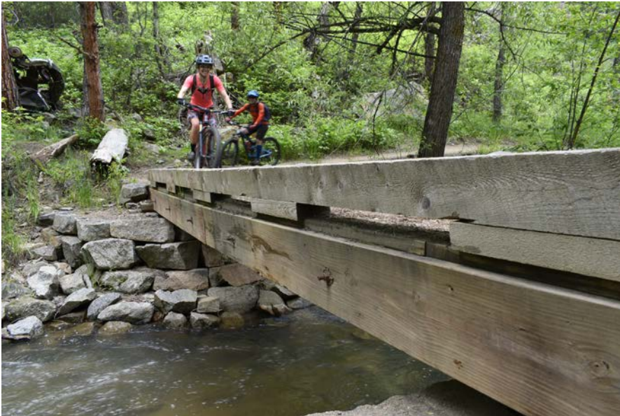
2023: The bridge has an obvious sag that developed in its first two years. Every long-span slab deck span sags to some degree. The longer the span and the thinner the slab, the more it sags.
