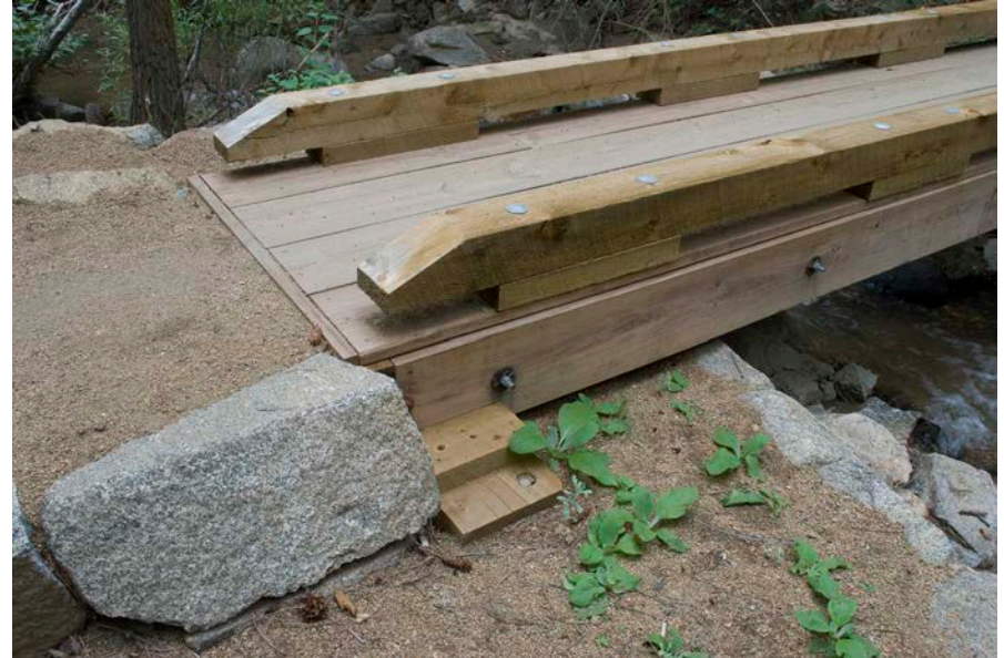
Note 2×6 block mounted on top of sill to keep the bridge from sliding sideways on the sill. These blocks are at all four corners. The span is not attached to the sills or the blocks. Note the tapered, elevated ends of the bull rails.
