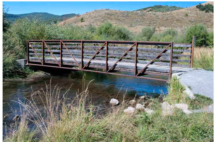
Both photos above: A weathering steel truss bridge on the Pony Express Trail in Utah softens its contemporary appearance and looks more historic by using softwood 2x6 mid-rails instead of standard thin steel mid-rails. It works; we process the bridge as being more naturalistic than we would with steel mid-rails.
