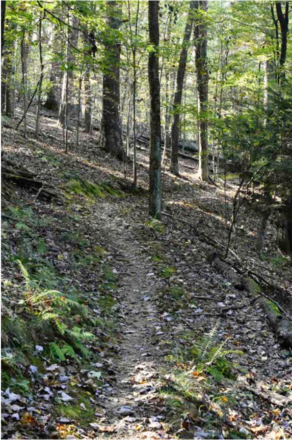
30-06 backslope is too steep and consequently slumped even on this gentle-moderate slope. Note slumping and narrowed tread in the immediate foreground. Good reversing grade.
