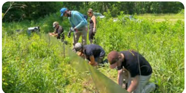
Students from The Ohio State University and West Liberty University construct a drift fence to direct wildlife towards cameras that document activity and biodiversity.
