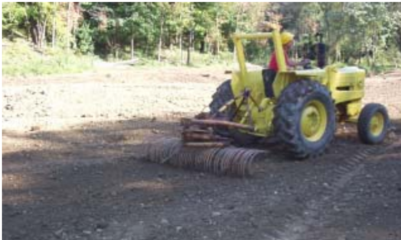
A major portion of work in the Chippewa Subdistrict in 2003 focused on improvements to Structure VII-D. Drainage improvements were part of the work as well as improvements along the structure itself.
