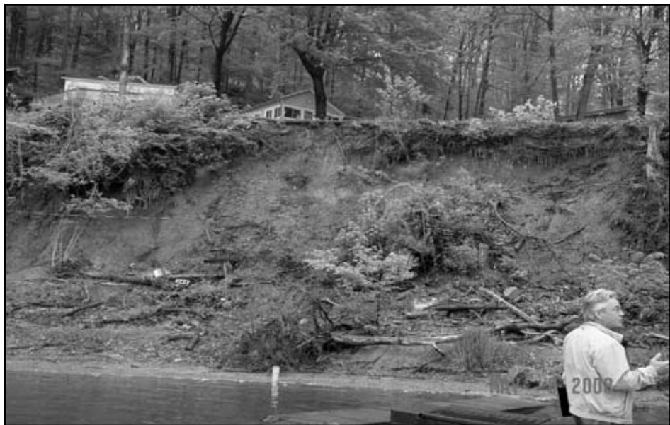
This section of shoreline at Pleasant Hill Reservoir has been identified as the top priority for stabilization by the MWCD in 2009. The MWCD staff also is reviewing the shorelines at all of its reservoirs for development of a plan to address erosion and stabilization issues.
