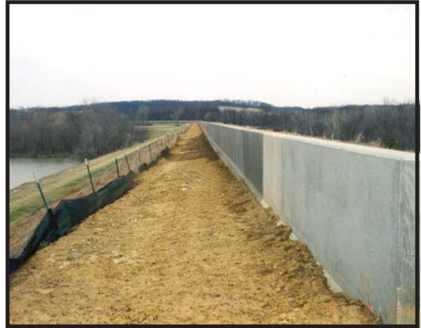
The USACE has embarked on a program to make improvements to its dams.
